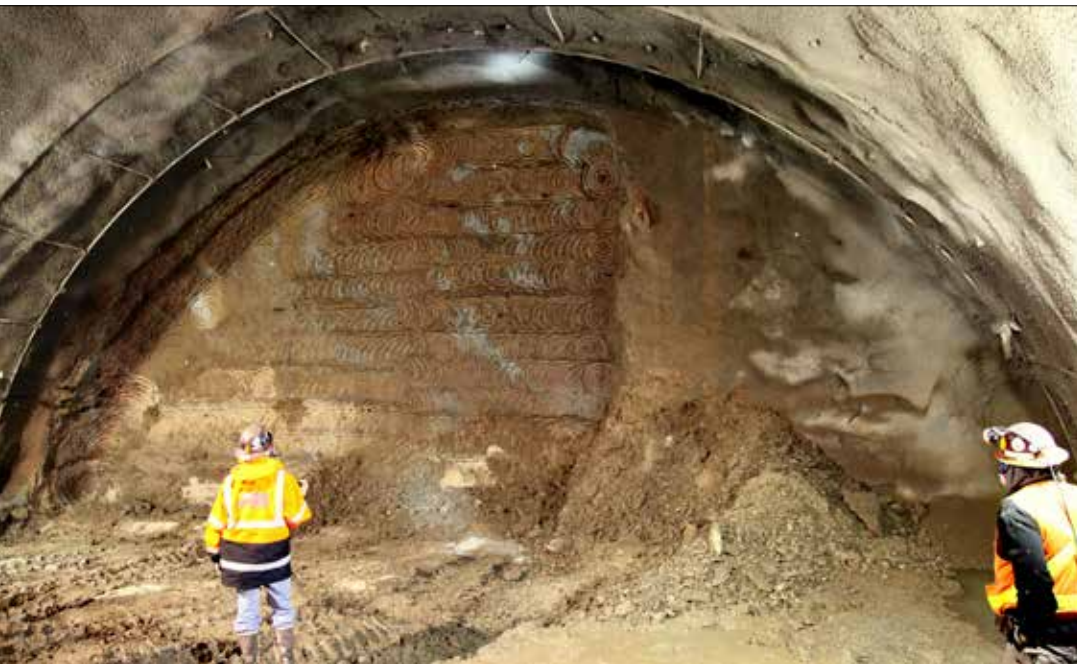
Top heading mapping in good ground – Caldecott Fourth Bore Tunnel. All article photographs by Sue Bednarz
