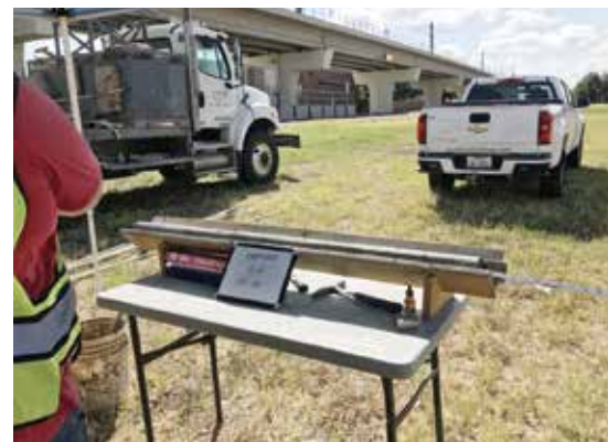
Careful geotechnical investigation and detailed analysis of the data were necessary for the redesigned tunnel alignment
