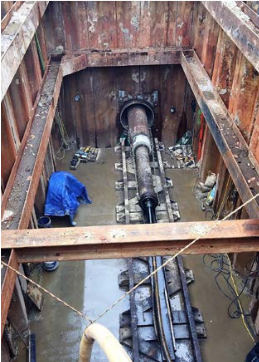
Figure 5. Taurus pipe ram driving a section of 24-in.-diameter casing. (Photo courtesy of Engineers Construction Inc.)
