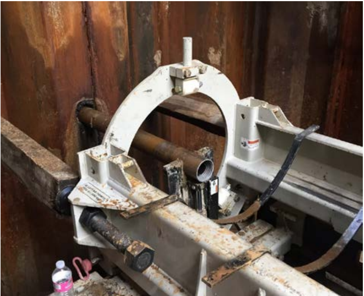
Figure 3. Pilot tube installed with an Akkerman head. (Photo courtesy of Ellingson Companies.)
