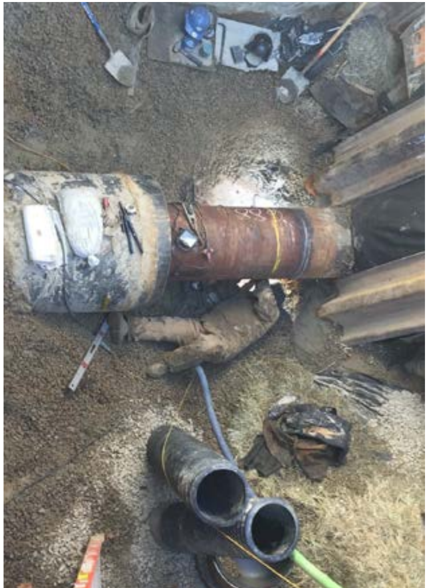
Figure 4. Welding an adapter to accommodate a transition between 24-in.- and 42-in.-diameter casings. (Photo courtesy of Engineers Construction, Inc.)
