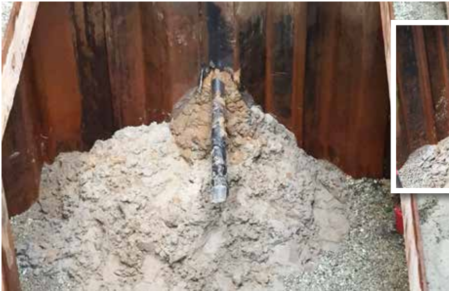
Saturated fine sand flowing into the receiving shaft.
