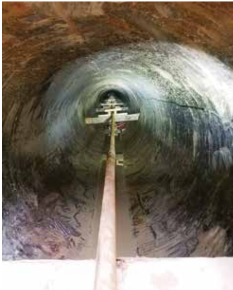
Pilot tube guidance system for the tunnel - Thinking out of the box.
