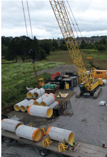
A shot of microtunneling work on the Stantec-designed York Downs Sanitary Sewer Connection project in Markham, Ontario. Courtesy of Stantec.
