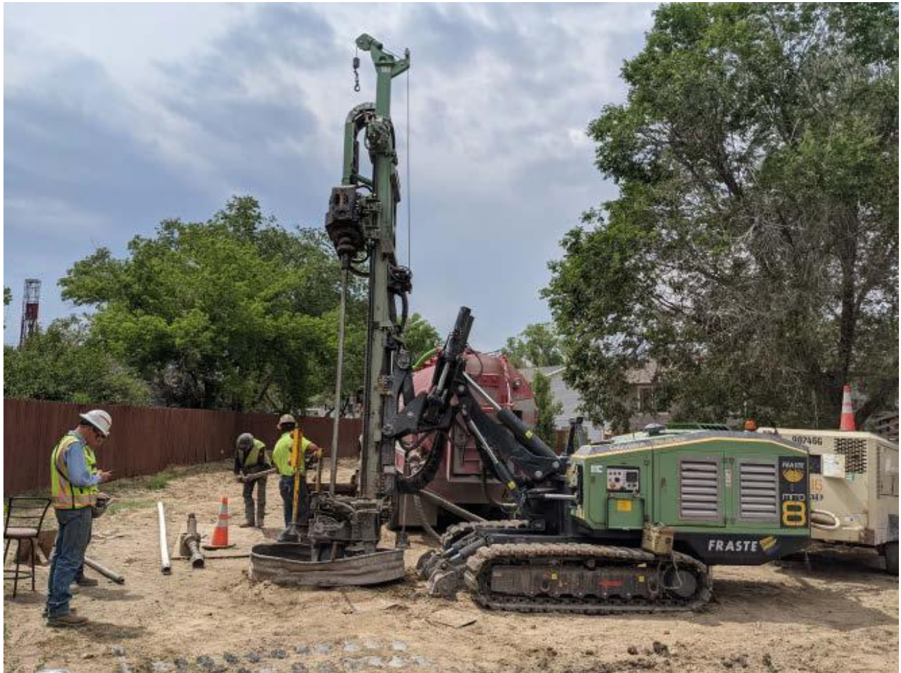
Figure 5. A geologist logs a borehole during an AML subsidence mitigation program using a mobile application for near real-time analysis by the construction manager.
