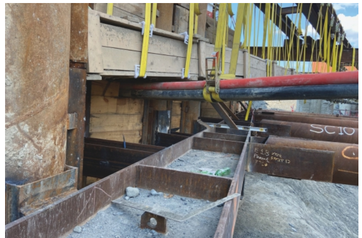
Close proximity of utilities and excavation support elements
